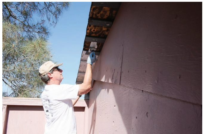
Caption: Roland Albers applies a sealant to underside of the roof. Credit: Ross Gaunt
