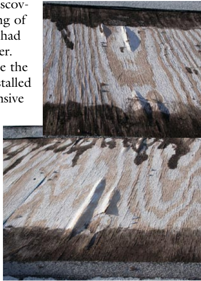
Close-up of the damage.
