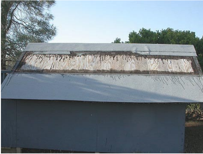
The damage to the roof is quite obvious. Photos: Ken Sperber
