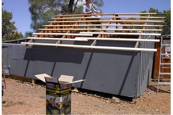
Removing the damaged roof gave us a well ventilated observatory, perfect for getting the scope cooled down quickly.
